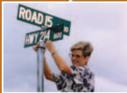
All county roads in the region were mapped, named and sign installation had begun. Parmer County Judge Bonnie Heald pictured with one of hundreds of signs installed in the region.
